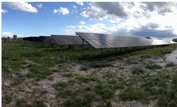
The photovoltaic facility in Gam in north-eastern Namibia’s Otjozondjupa region is currently the country’s largest off-grid hybrid energy system.
