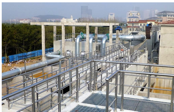
Biofiltration plant at a Chinese municipal wastewater treatment plant.
