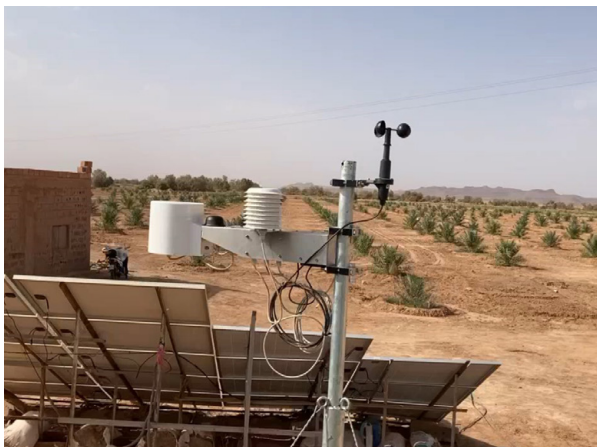
PV powered irrigation and weather station in Errachidia.
