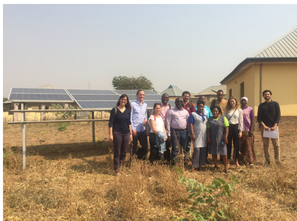
Solar system Dakwa PHC.
