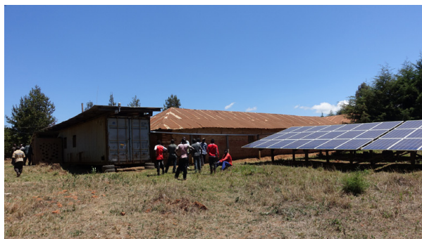
GridsPower supply with solar systems.
