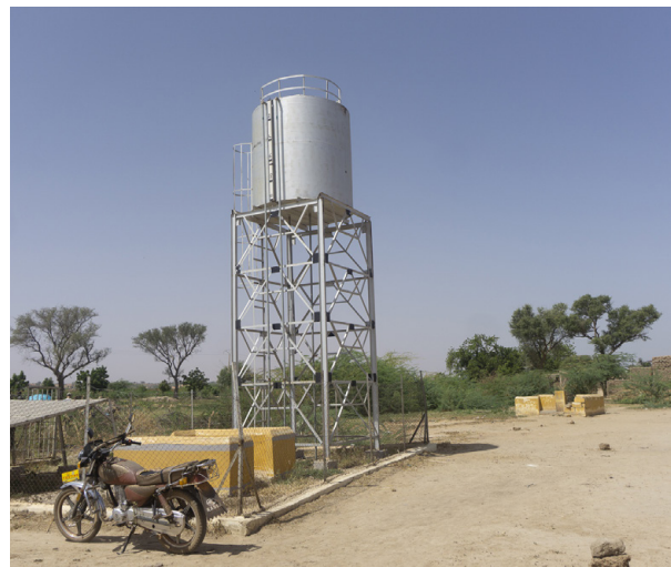
Solar water pumps in Niger.
