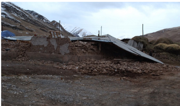
A building in Kyrgyzstan destroyed by the magnitude 6.8 Nura earthquake.
