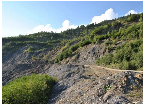
The “Black Channel” on the road towards Mestia in the Enguri river valley.
