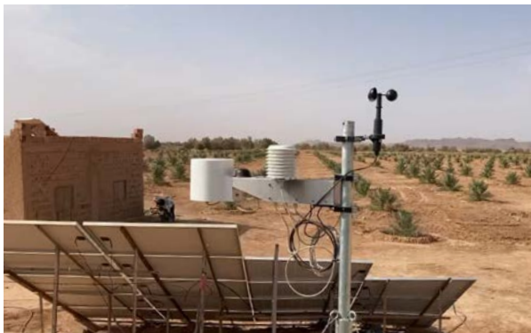
PV powered irrigation and weather station in Errachidia.
