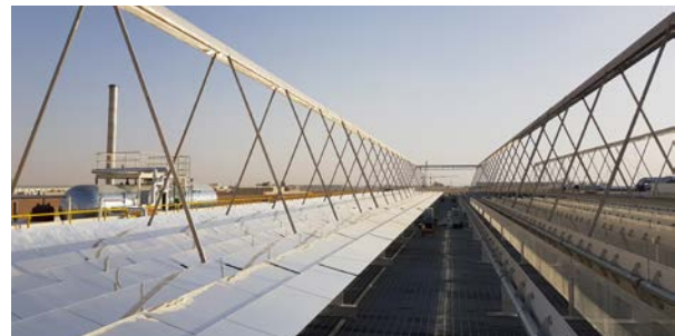
Solar thermal energy on the roof of an industrial plant.
